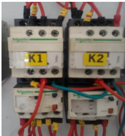
Figure. 8. Contactor and Thermal overload
